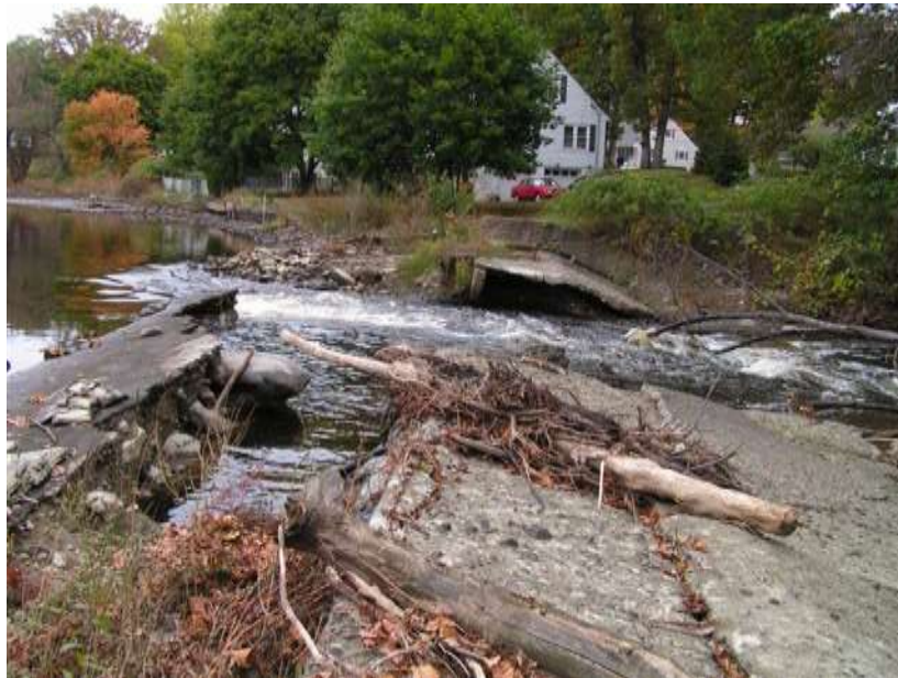
Figure 7.4 Damage to Winona Lake Spillway in Orange County on Quassaick Creek.
