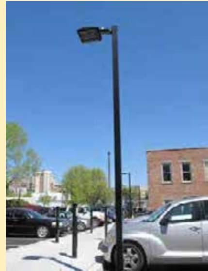
Efficient LED lights have been installed in the Library South parking lot.
