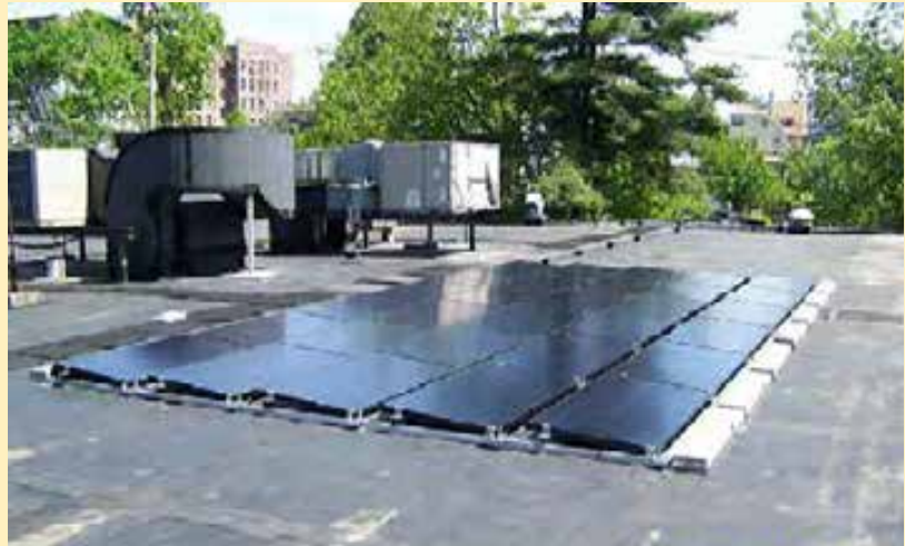
Solar panels have been installed at the Hugh Doyle Senior Center.
